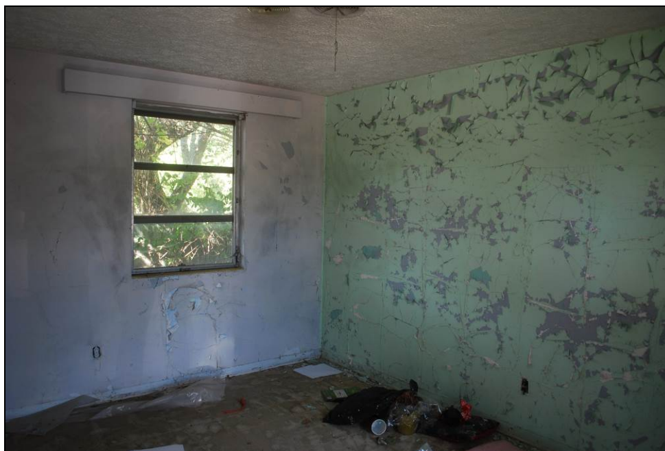
Photograph 14. Interior of a Unit and Teal Wall Coloring, Building No. 2
